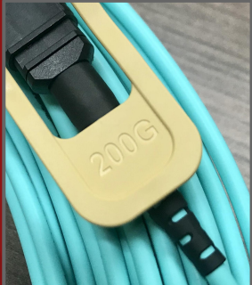
HDR fiber cable used to connect Fir to Sherlock HDR LNet routers
